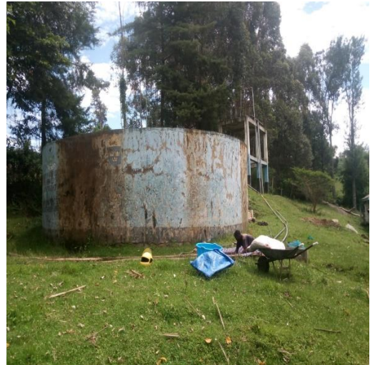
Figure 1: Kimng'oror water plant - water reservoir
